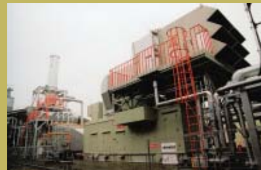
Cogeneration system at the Mishima Plant.
