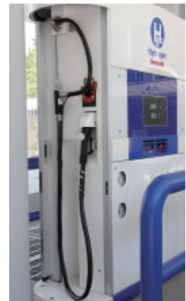
A Yokohama hose at a hydrogen filling station
