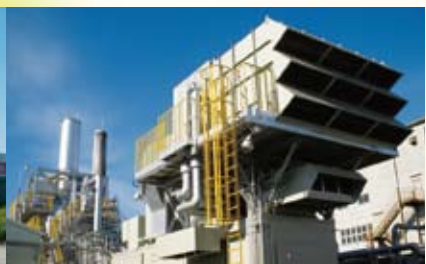
A cogeneration system at our Shinshiro Plant, in Japan
