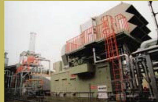
Cogeneration system at the Mishima Plant.
